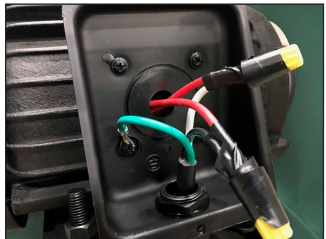
Figure 73. G1033X motor junction box.
