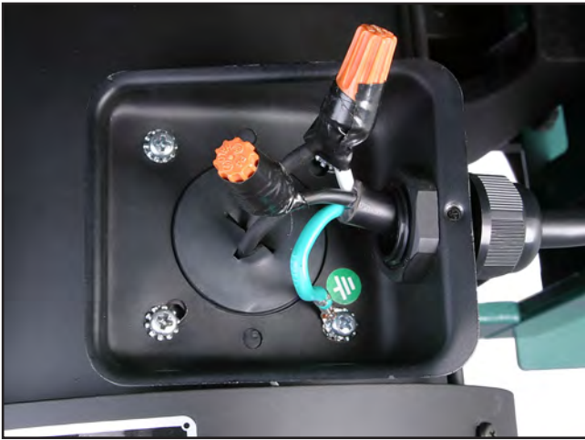
Figure 84. G0605X motor junction box.
