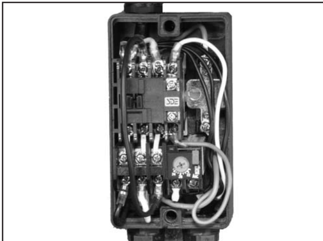
Figure 4. 220V Magnetic Switch
