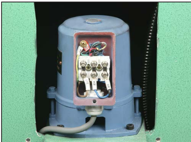
Figure 78. Pump motor (M2) connections.
