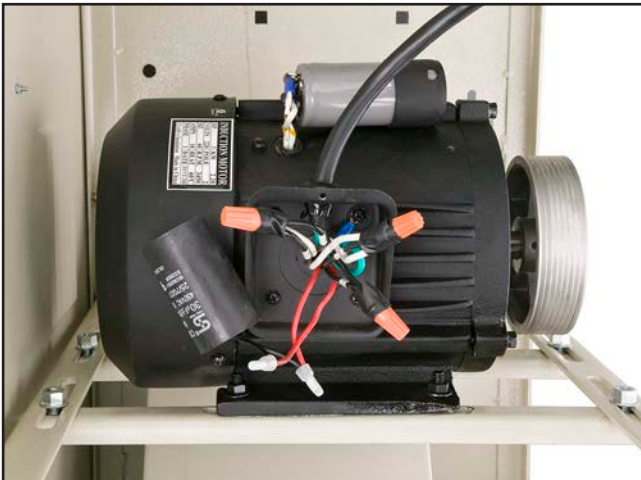
Figure 68. Motor and capacitors.
